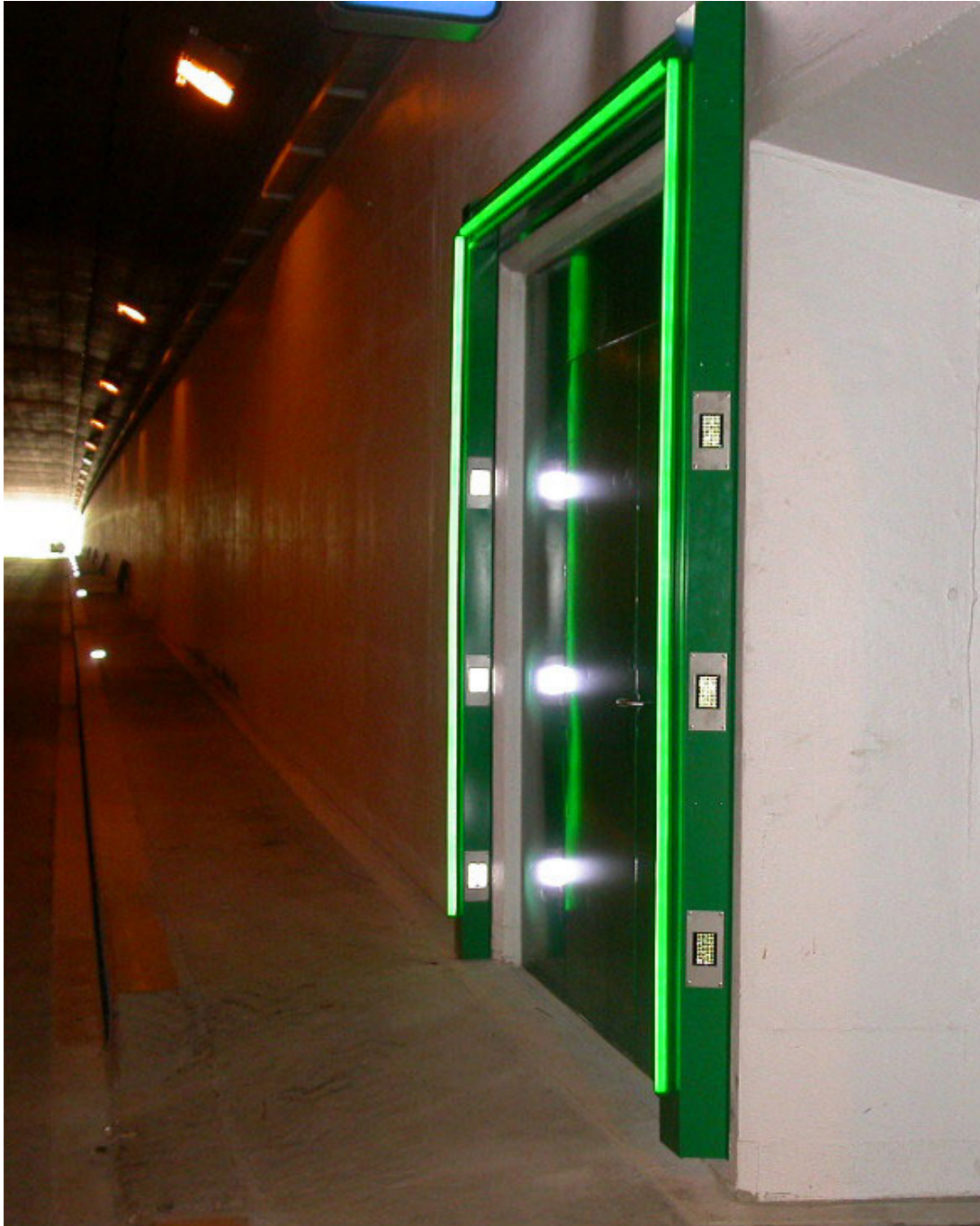
Emergency exit in road tunnel
